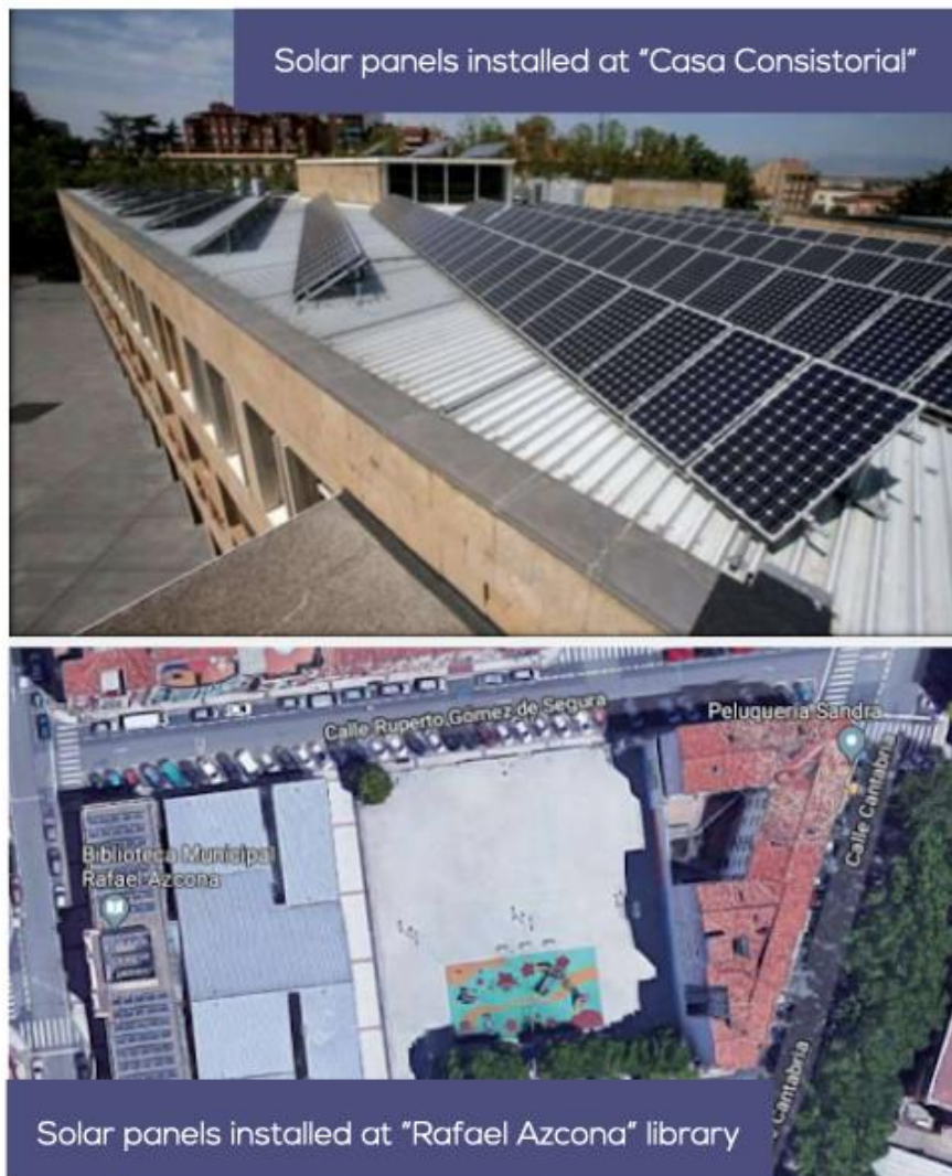
Figure 3. Solar panels installed in municipal buildings
