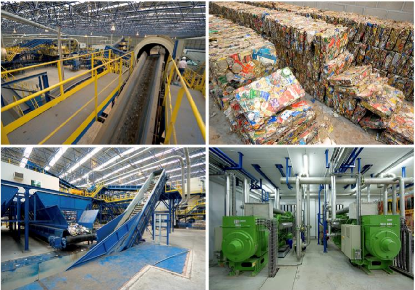
Figure 1. Ecoparque: waste treatment facility of La Rioja
